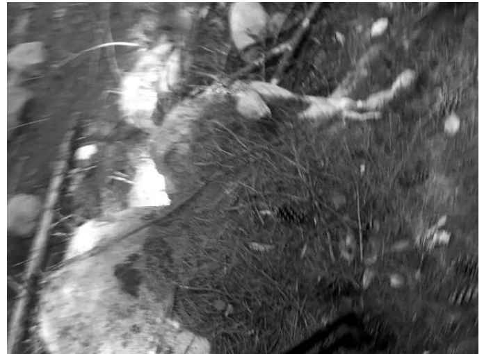
Washout in wall very little missing · 22 Jul 2019
